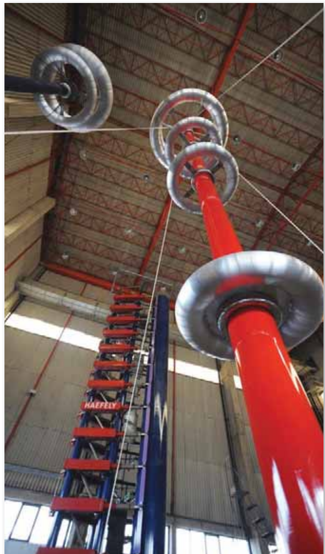
Lightning impulse generator voltage divider.
